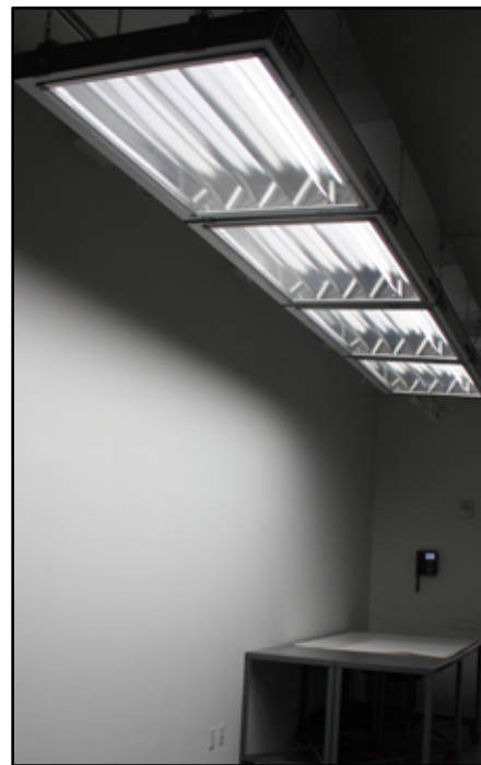
VS + Company's primary viewing area includes four GTI GLE-532A overhead luminaires.
