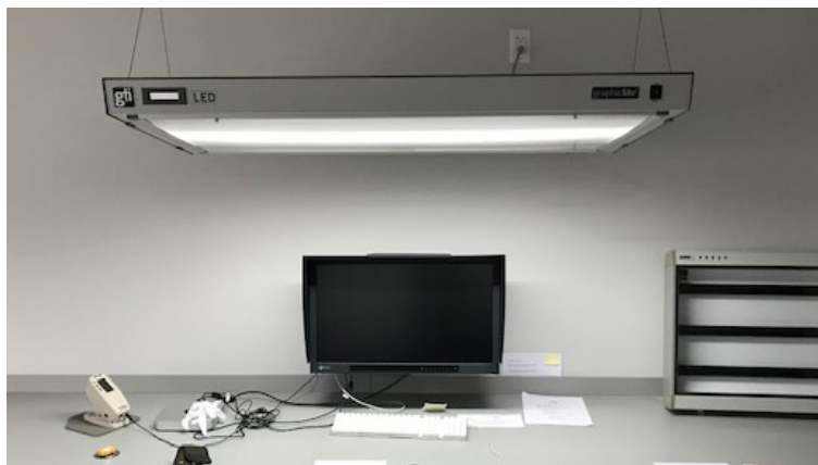
GTI's GLE-348A/LED/SP luminaire installed at Meredith Corporation's headquarters in Des Moines, IA.
