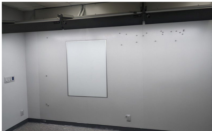
Circle Graphics uses three GTI GLL-548/LED/V wall viewing luminaires to create a vertical viewing that is 12' long x 8' tall.
